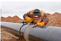
Operation of Pipelines
